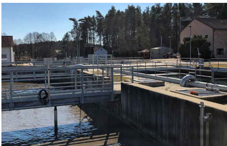
Fig. 1: View of Sewage treatment plant Hilpoltstein
