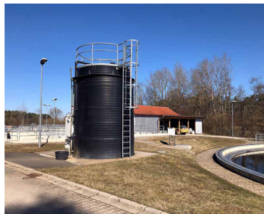
Fig. 2: Precipitant tank at the Hilpoltstein wastewater treatment plant with Alyza IQ PO 4 (next to it on the right).
