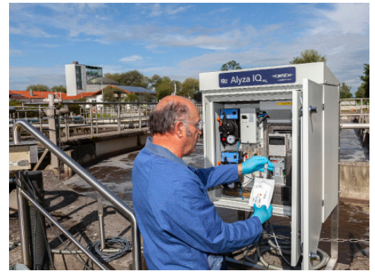
Figure 6: The Alyza IQ PO 4 at the Weilheim wastewater treatment plant
